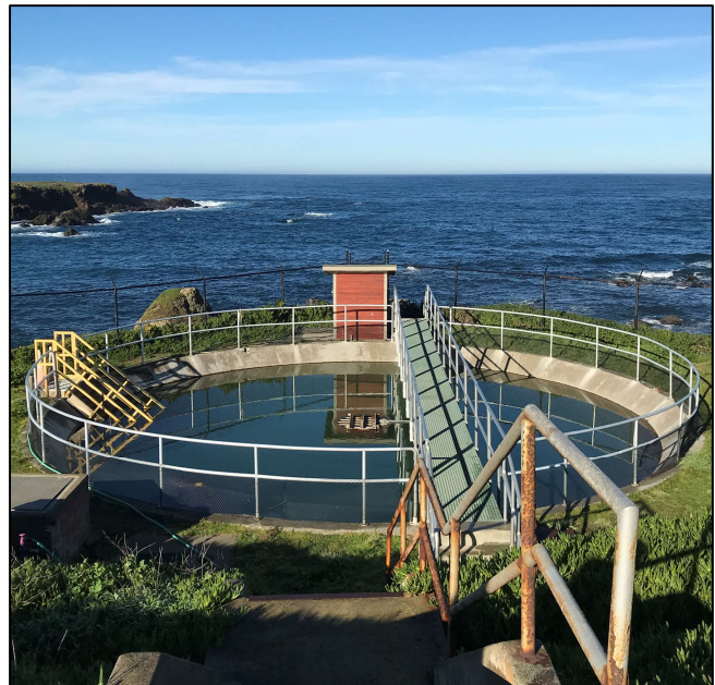
View west to Pacific Ocean where the new intake would be located. Foreground shows the existing outfall infrastructure where discharge would be tied in.
