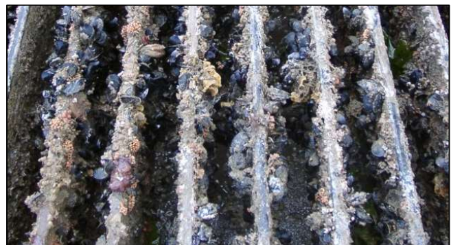
Trash rack bars fouled with various organisms (courtesy Pecten Aquatic)
